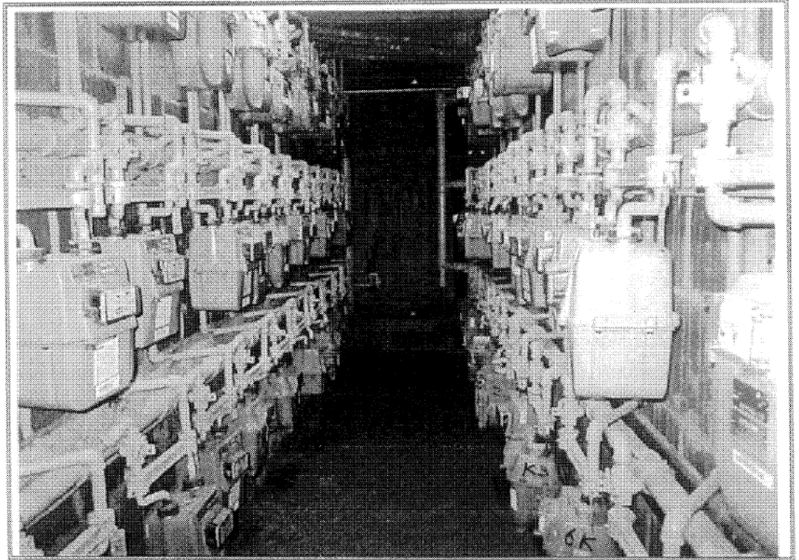
View of the gas meters
