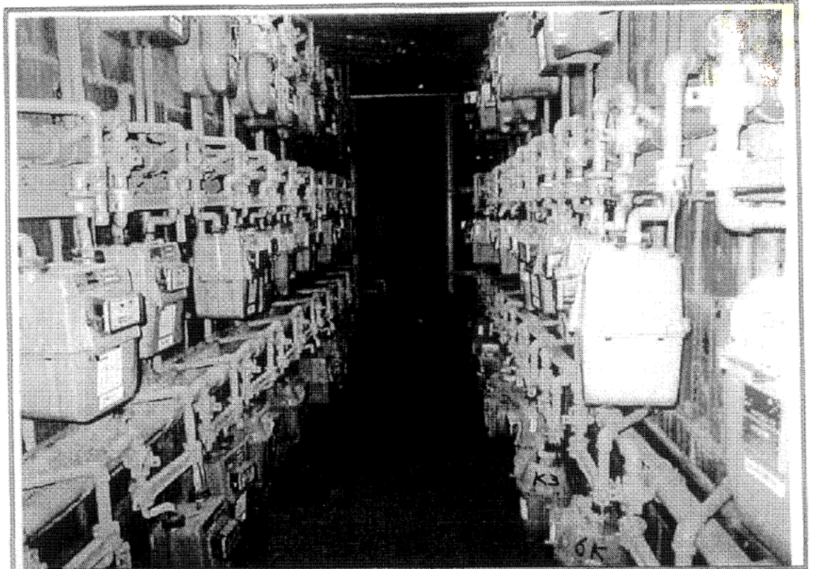
View of the gas meters
