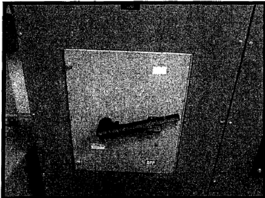
Figure 2.3.5 – Main Service Disconnect.
