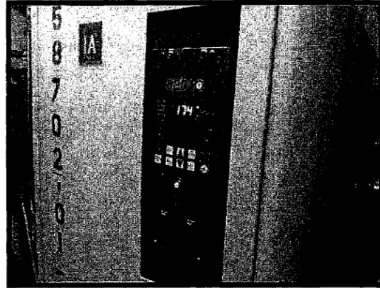
Figure 2.4.12 – Hot Water Boiler.
