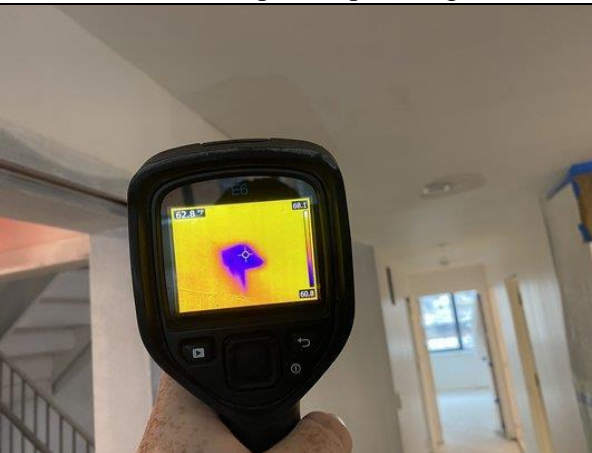
Additional recent spackle patching; moisture content is locally elevated but surrounding materials are dry (<150 REL)
