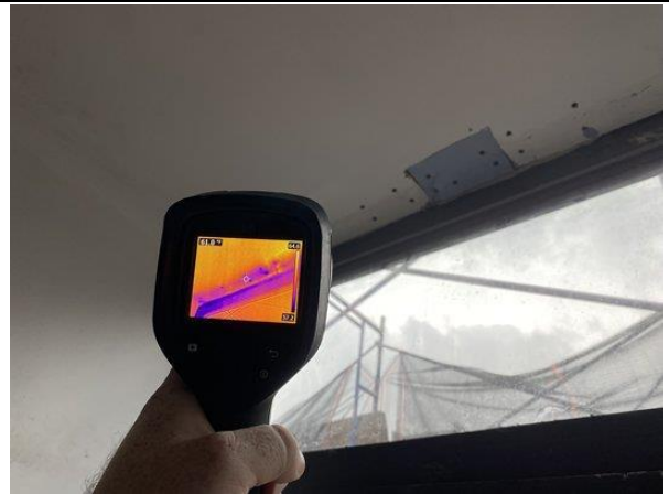
Thermal bridging observed on stained window soffit
