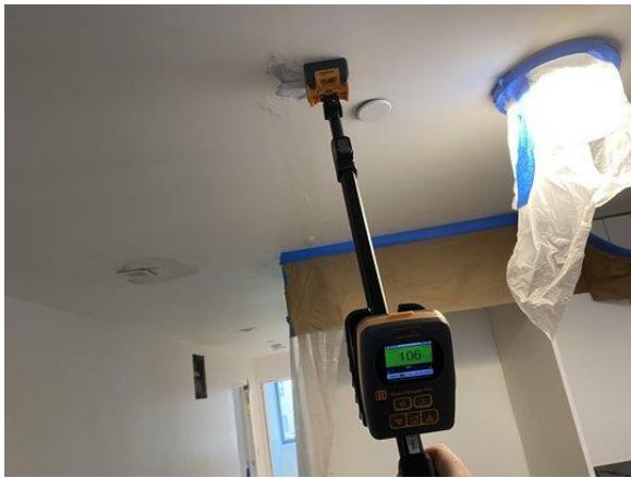
Thermal bridging from concrete substrate verified via moisture meter
