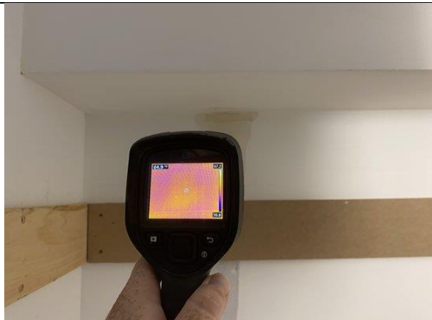
Water damage in 6h floor primary bedroom walk-in closet is dry with no EMC or remaining surrounding damages
