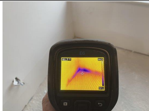
Typical minor local elevated moisture content remaining in recently spackled walls; higher moisture content is observed in areas with heavier application of the compound
