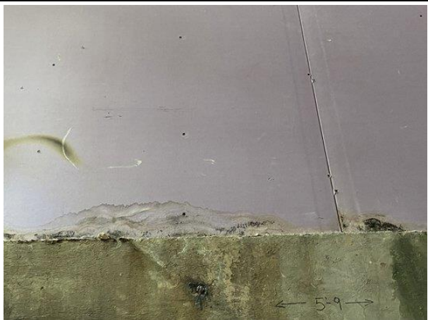
Water damage observed at 6 th floor unit roof bulkhead (<3 SF)
