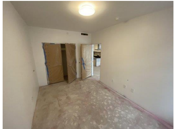
Typical Bedroom 3 layout at the SW corner from Floor 5 through 2; normal findings
