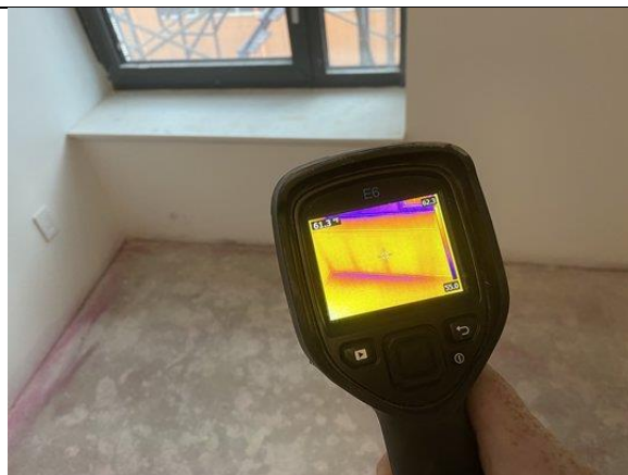
Typical thermal bridging observed in South facing walls adjacent to the curtain wall system
