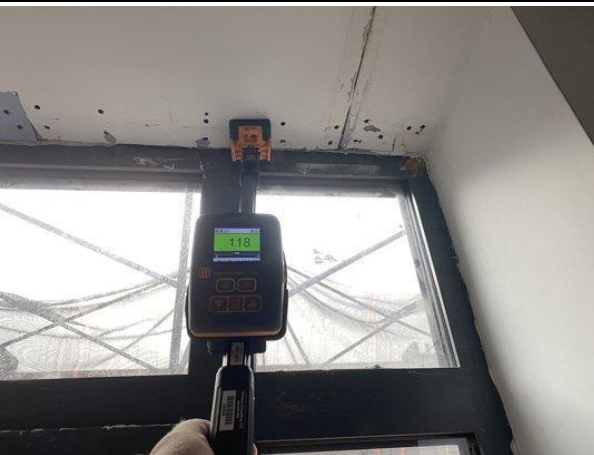
Normal moisture content reading on stained gypsum awaiting refinishing
