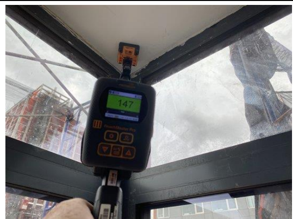
Normal moisture content in areas with minor temp variation and visible discoloration from spackle
