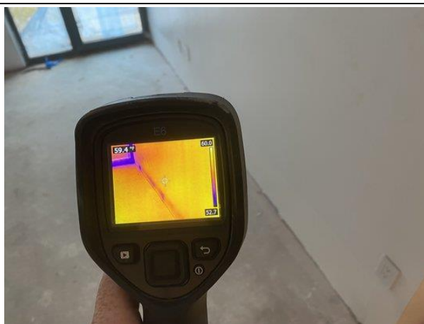
Typical EMC on patching in primary NW bedroom; representative of floors 5 through 2
