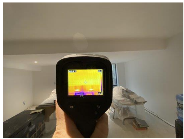
IR view of the 1 st Floor unit's rear cellar space; normal findings
