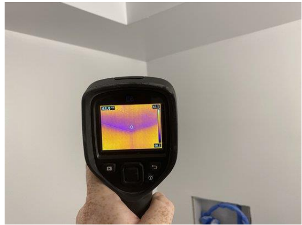
Minor temperature differential in NE bedroom 2 soffit
