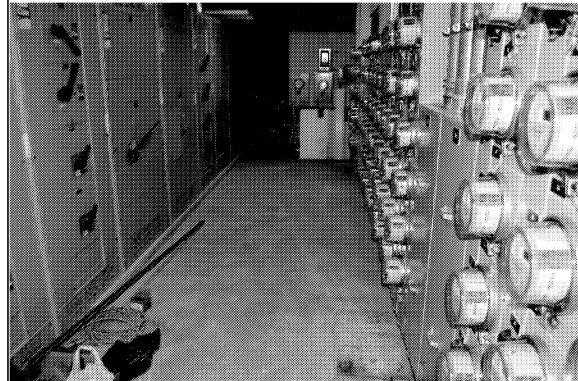
Photo #22: Electrical system
