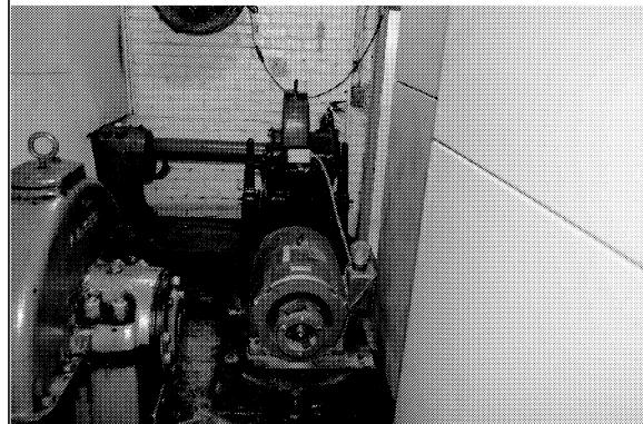
Photo #24: Typical elevator machinery
