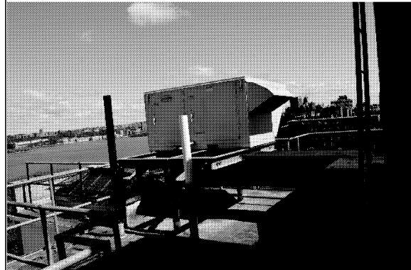
Photo #10: Typical RTU
