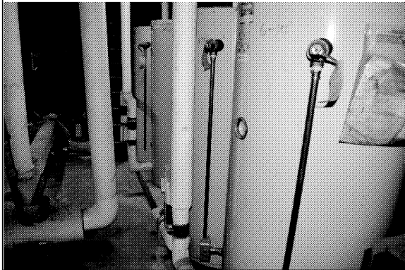
Photo #19: Indirect water heaters
