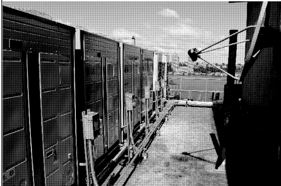
Photo #9: VRF condenser units on roof
