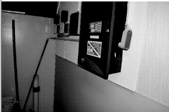
Photo #23: Fire alarm panel
