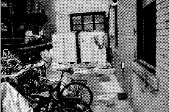
Photo #27: Amenity space condenser units
